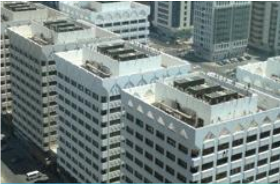
Roof Top Chillers
